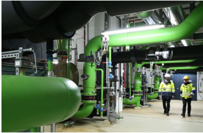
Generating heat from cold for city buildings
