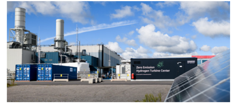
Zero Emission Hydrogen Turbine Center, Finspang, Sweden
